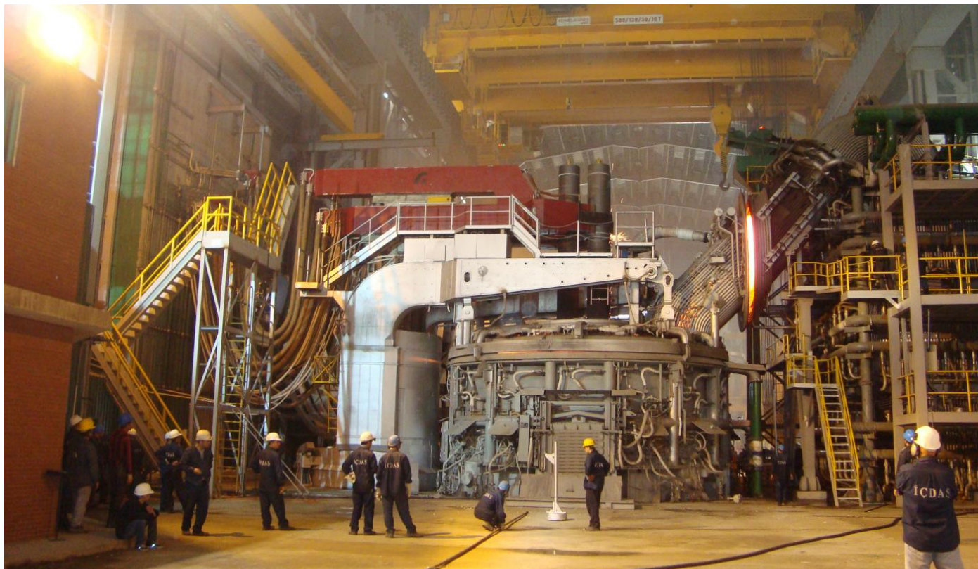
土耳其 220t 电弧炉热试 Hot test of 220t electric arc furnace in Turkey
