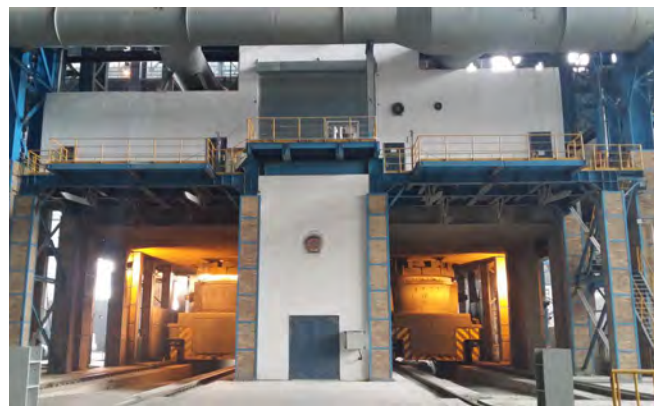
日照工厂 300t 精炼炉 300t refining furnace in Rizhao
