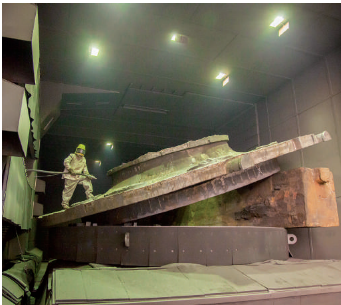
The critical surface areas of very complex work pieces can be manually spot treated with a specially installed pressure blasting system.
