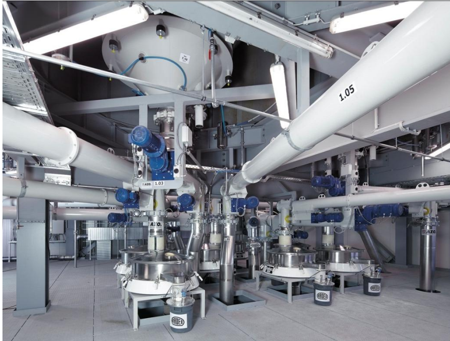
Dosing screws with screeners below
