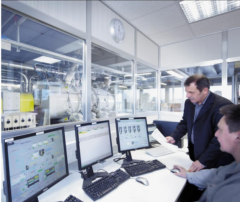
Control centre for operating and monitoring
