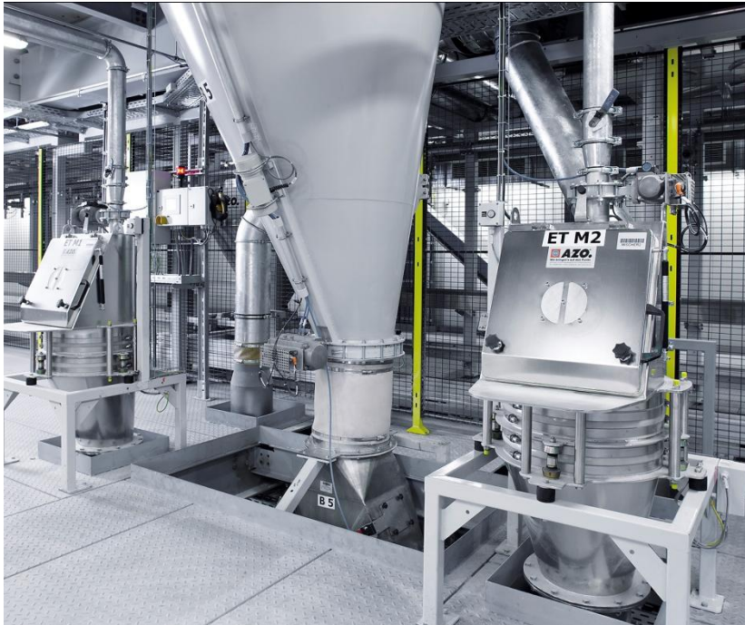
Feeding hopper for manual feeding directly into the mixer
