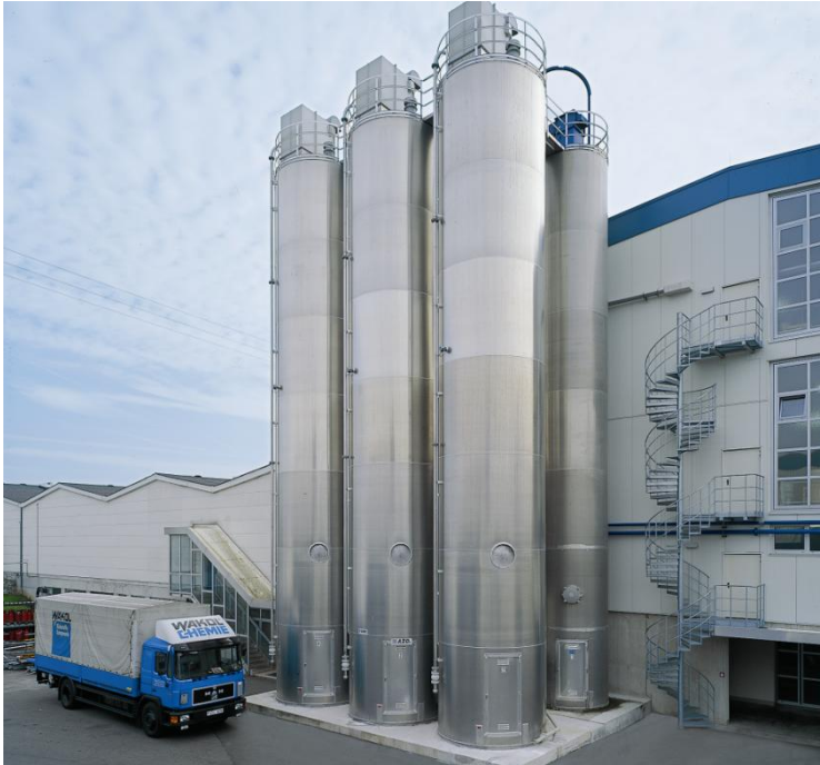
Outdoor silo with filling lines and filters
