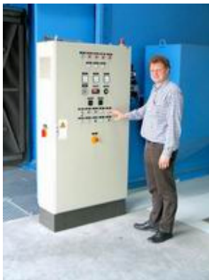
Foundry engineer Dr. Georg Dieckhues at the control panel of the AGTOS blasting unit.
